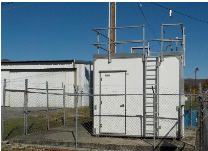
Figure 69: Middlesboro Air Monitoring Shelter
